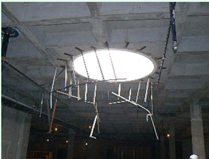
This skylight is where the old McHenry Library's signature spiral staircase was located. Though loved by many it was a fire hazard and had to go.
